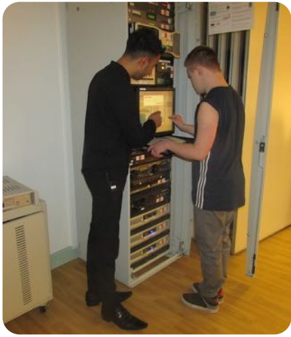
LUCAS PROGRAMMING THE 4D HALL EQUIPMENT WITH LYNX THE IT TECHNICIAN
